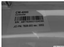
Label on Controller
